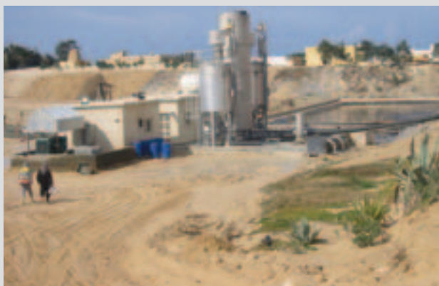
Gas flaring system for the project
