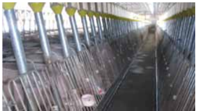
The Marcela Farms in the Philippines captures methane from manure and turns it into electricity and uses treated sludge as fertilizer for a banana plantation.
