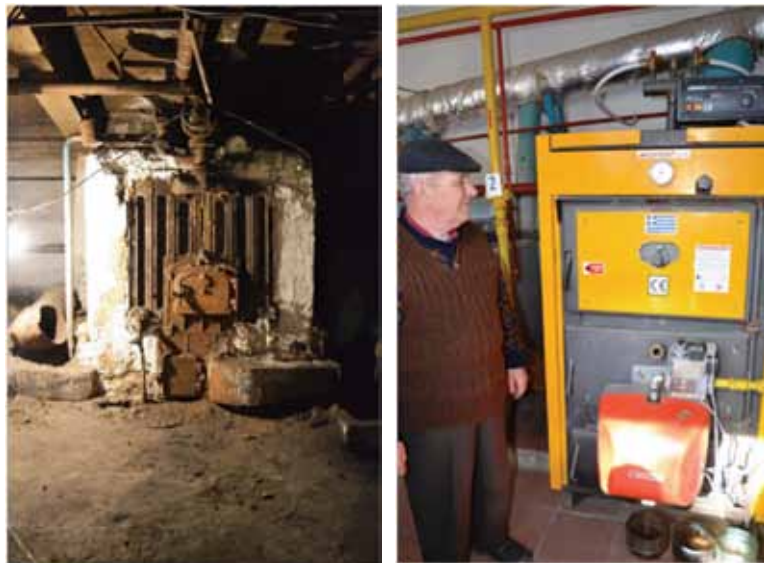
Before and After: New, efficient and programmable gas boiler heater versus inefficient Soviet coal boiler heater.
